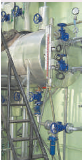
MBSK installé en chaufferie MBSK installed in boiler house
